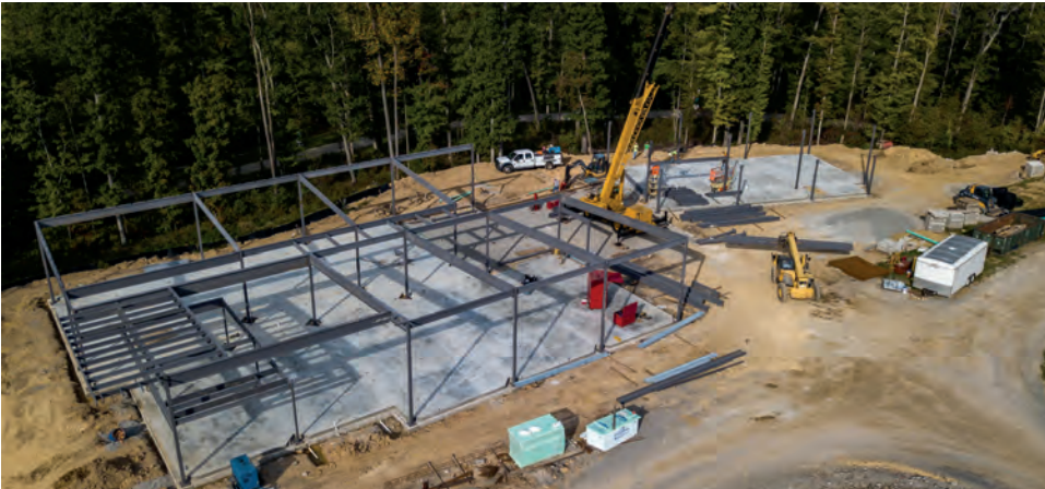
One of two leadership centers currently under construction at the Summit Bechtel Reserve, the Rex W. Tillerson Leadership Center will be a major component of the BSA's flagship ethics and leadership campus – the Thomas S. Monson Leadership Excellence Complex. Photo courtesy of the BSA.
